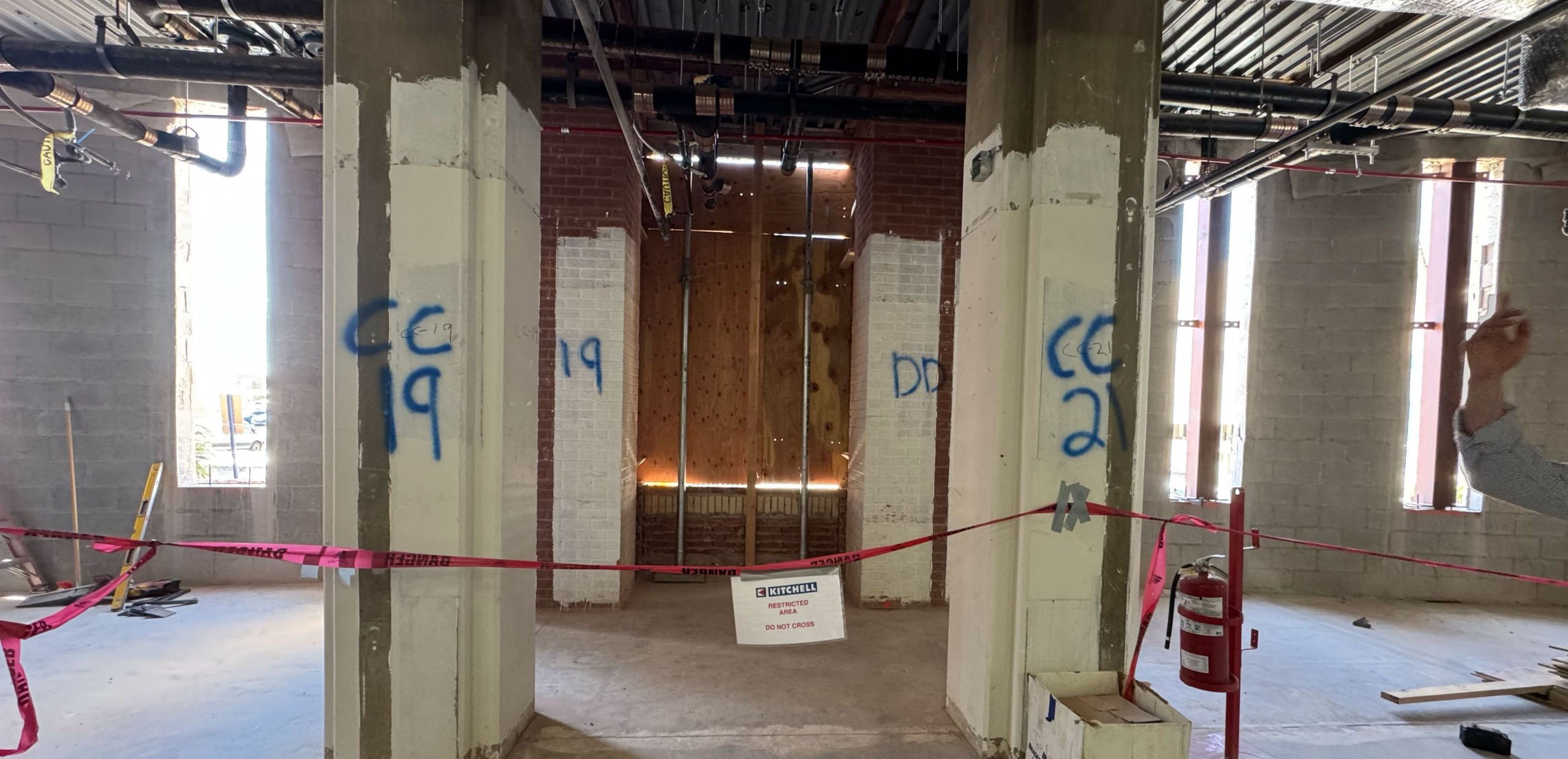
Updated Construction Progress: More Photos of Our New Home in the Making | March 2025
